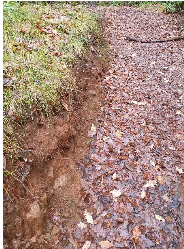
Figure 12: Image of root damage due to path construction.
